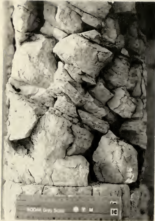
Fig. 19. Irregular and diagonal cracking of volcanic tuff blocks at intersection of west wall of nave and transept (Photo: Anne Brackin).
